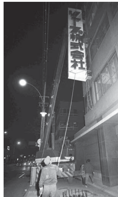
Replacing the outdoor signage of the head office reflecting the company's name change
